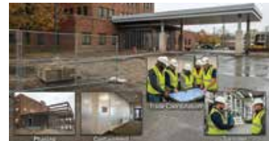
SYSTEMS COORDINATION Electrical, lighting, HVAC via licensed partners
